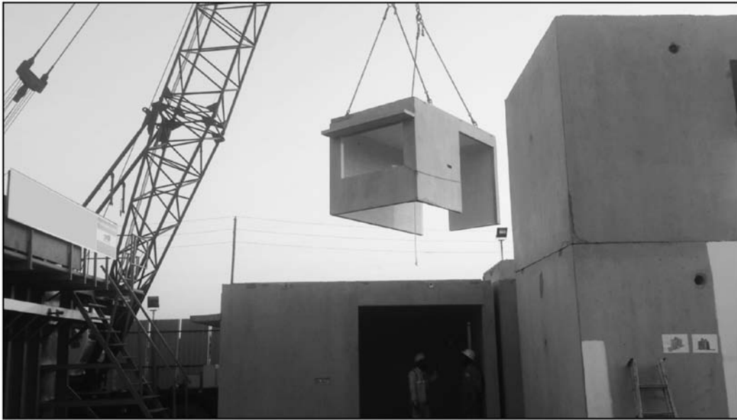
Figure 6. A 20-apartments five-storey building under construction using 3D Monolithic Shearwall Technology. The project was cast and installed in 33 days at Tata New Haven, Boisar-II, Mumbai. A two-month long testing of the building structure, connections, joints including leakage and seepage tests was successful.
